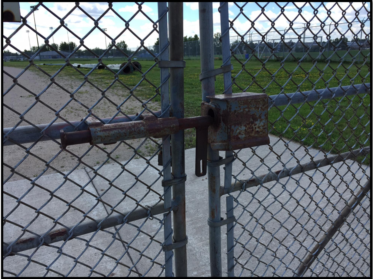
September 11, 2015 Wilkes Reservoir North Cell Rehabilitation Construction of Laydown Area 711-2015 Addendum 1 Tamper Proof Locking Mechanism at Existing North Gate of Reservoir
