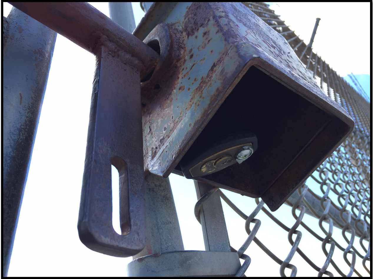
September 11, 2015 Wilkes Reservoir North Cell Rehabilitation Construction of Laydown Area 711-2015 Addendum 1 Tamper Proof Locking Mechanism at Existing North Gate of Reservoir
